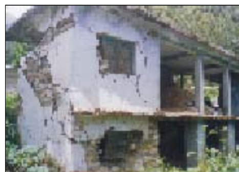
Fig. 2. Modern house damaged due to earthquake
